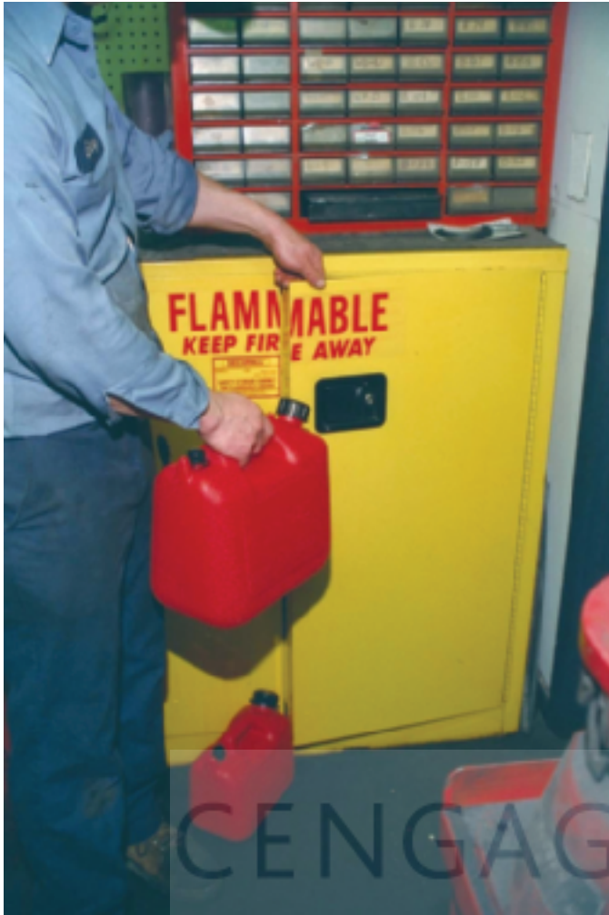
FIGURE 1-15 Chemical storage cabinets must be labeled as to contents and fire hazards.
